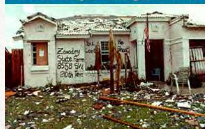
Level 3 - Major damage; uninhabitable
